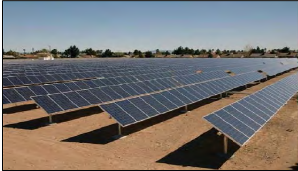
Photo 1. Typical Fixed-Tilt PV Panels
