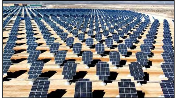
Photo 2. Typical Single-Access Tracking PV Panels
