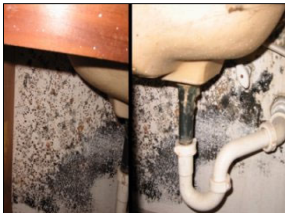
Mold on drywall under leaky sink
