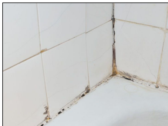
Mildew found on bathroom grout
