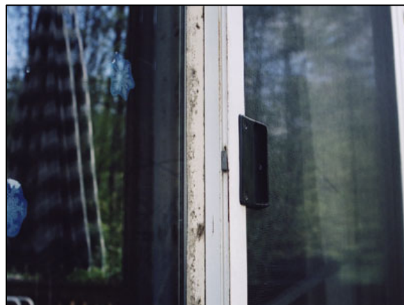
Mold on air seal on sliding glass door
