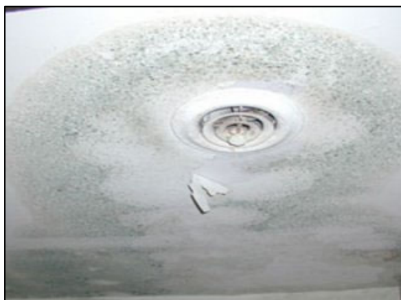
Mold surrounding air conditioning vent
