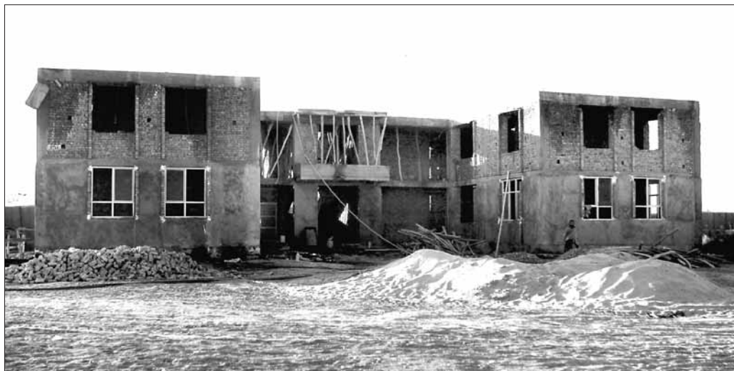
The Nawa, Afghanistan's District Governance Center was under construction in December of 2009. The war-torn structure has been transformed from a makeshift military patrol base into a functioning building which will house government offices for Nawa District.
