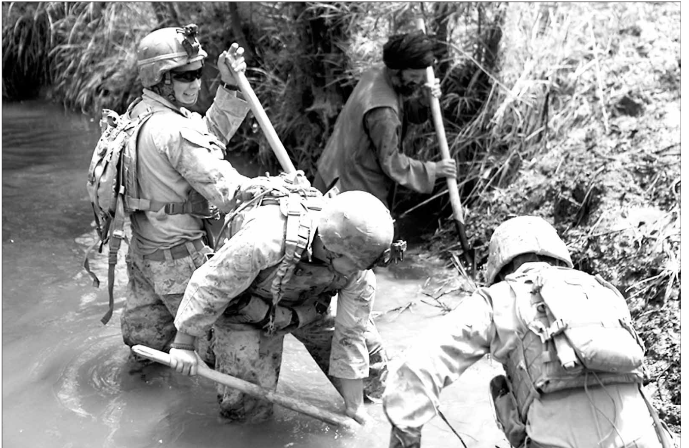
Marines with Company K, 3rd Battalion, 7th Marine Regiment, shovel mud and obstacles out of a canal, July 30. Marines, Afghan soldiers, and locals all helped repair two canals in the area.
