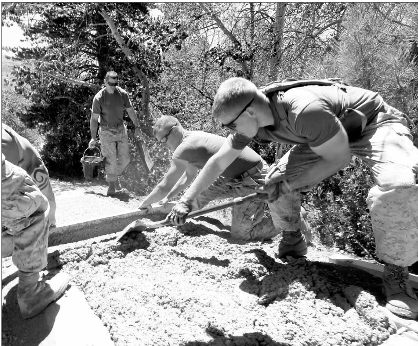
Combat Engineers with Company C, 3rd Engineer Support Battalion, spread concrete for a 500-foot sidewalk at the Marine Corps Mountain Warfare Training Center July 26.
