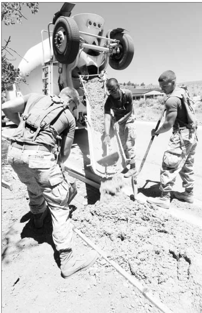
Marines with Co. C, 3rd CEB, guide concrete from a cement mixer onto their wooden construction grids.
