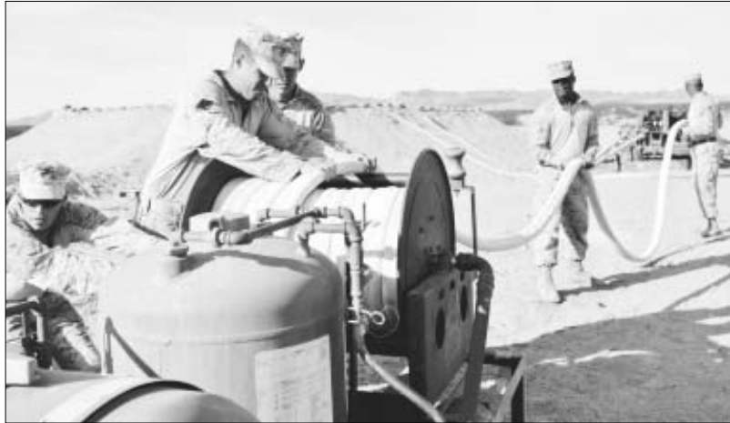
Marines with Engineer Company retract a fire hose after an immediate action drill at Marine Air Ground Combat Center Twentynine Palms, Calif., Dec. 2, where they responded to a simulated fire in one of the fuel reservoirs on a forward fuel farm they established during Enhanced Mojave Viper. In the event of a real incident, the Marines would be called upon to contain and extinguish the fire before it jeopardizes the functionality of the fuel farm. Engineer Co. is attached to Combat Logistics Battalion 4, Combat Logistics Regiment 3, 3rd Marine Logistics Group, III Marine Expeditionary Force.
