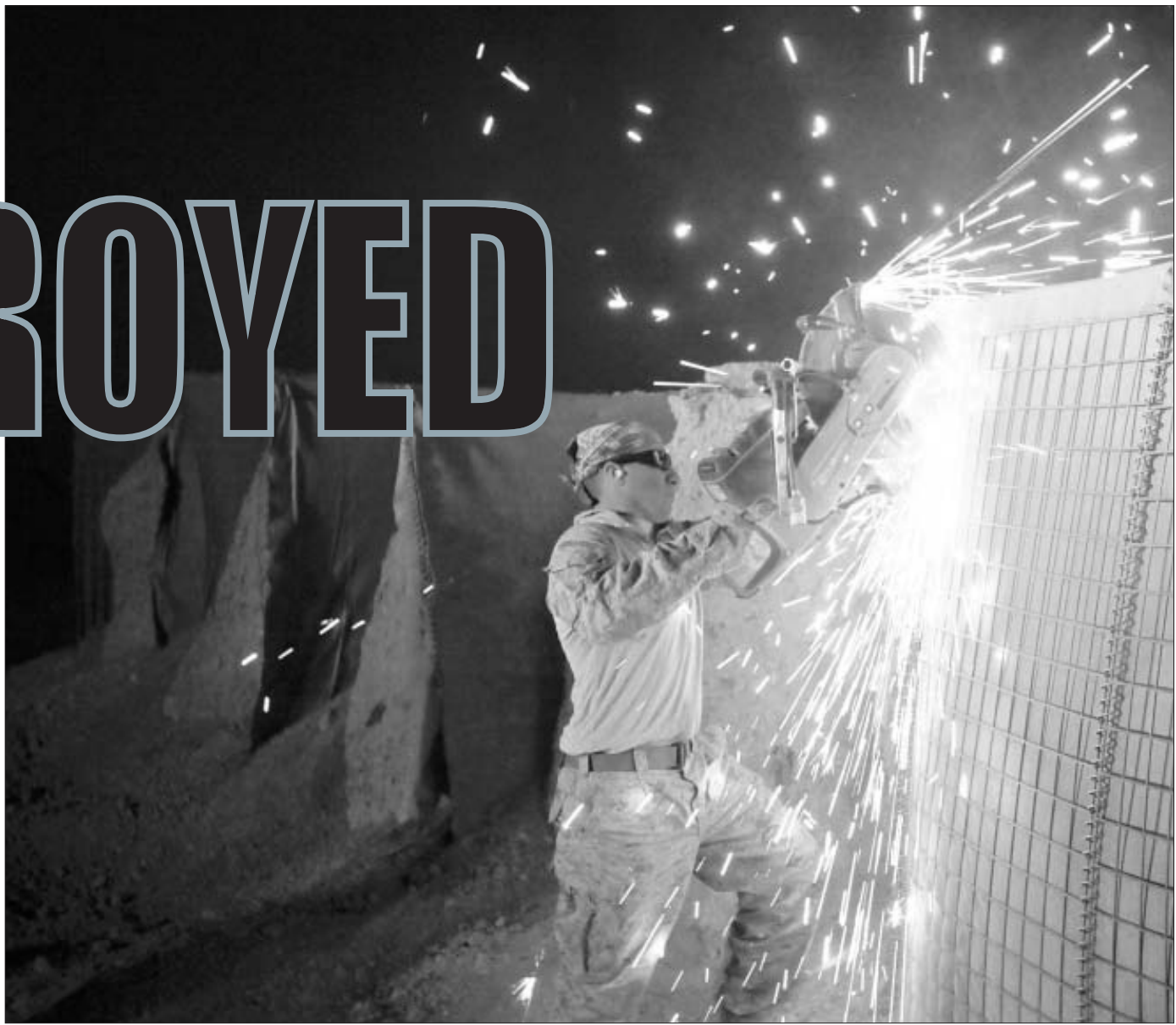
Cpl. James Hernandez, combat engineer with Company A, 9th Engineer Support Battalion, uses an electric saw to dismantle a dirt-filled barrier at Firebase Saenz Dec. 13.
