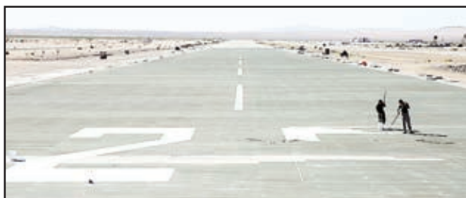
Cpl. Jeremy Montoya, crew leader, Marine Wing Support Squadron 374, and Sgt. Horacio Leyva, Runway supervisor, MWSS 374, paint numbers on the approach section of the Strategic Expeditionary Landing Field at Camp Wilson, Monday. The Marines were involved in a 2,000-ft. matting project at the SELF.
