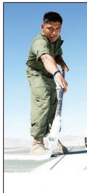
Sgt. Horacio Leyva, runway supervisor, Marine Wing Support Squadron 374, paints the number at the approach section of the Strategic Expeditionary Landing Field, Camp Wilson, Monday. The section was replaced to make the approach safer for aircraft that land at Camp Wilson.
