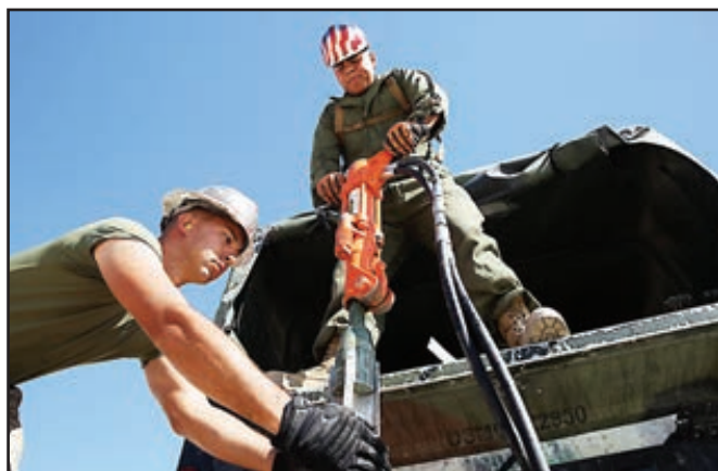
Lance Cpl. Romen Hines, crew member, Marine Wing Support Squadron 374, and Lance Cpl. Timothy Sakaida, crew member, MWSS 374, jackhammer stakes to anchor panels into the ground at the Strategic Expeditionary Landing Field, Camp Wilson, Monday.
