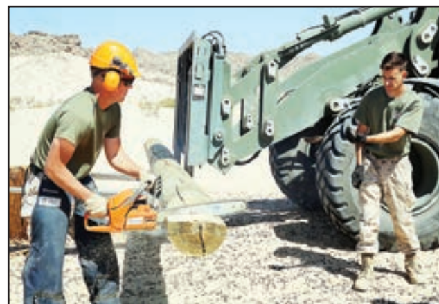
Cpl. William Hamilton, combat engineer, Combat Logistics Battalion 7, takes direction from Cpl. Corey Worobi, combat engineer, CLB-7 while sawing a log during the renovation of the obstacle course near the East Gym, Sept. 29. The use of Marines for the project is expected to save the government approximately $50,000.
