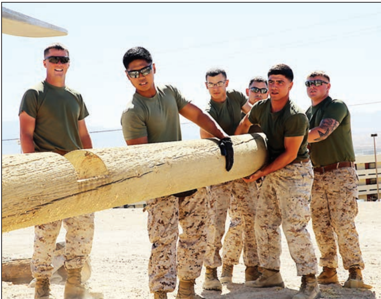
Marines with Combat Logistics Battalion 7 work together to lift a log during the renovation of an obstacle course near the East Gym, Sept. 29.
