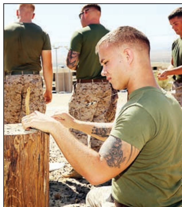
Cpl. Brandon Wilson, combat engineer, Combat Logistics Battalion 7, levels a post during the renovation of an obstacle course by the East Gym, Sept. 29. The project began two weeks ago and is expected to end sometime next month.
