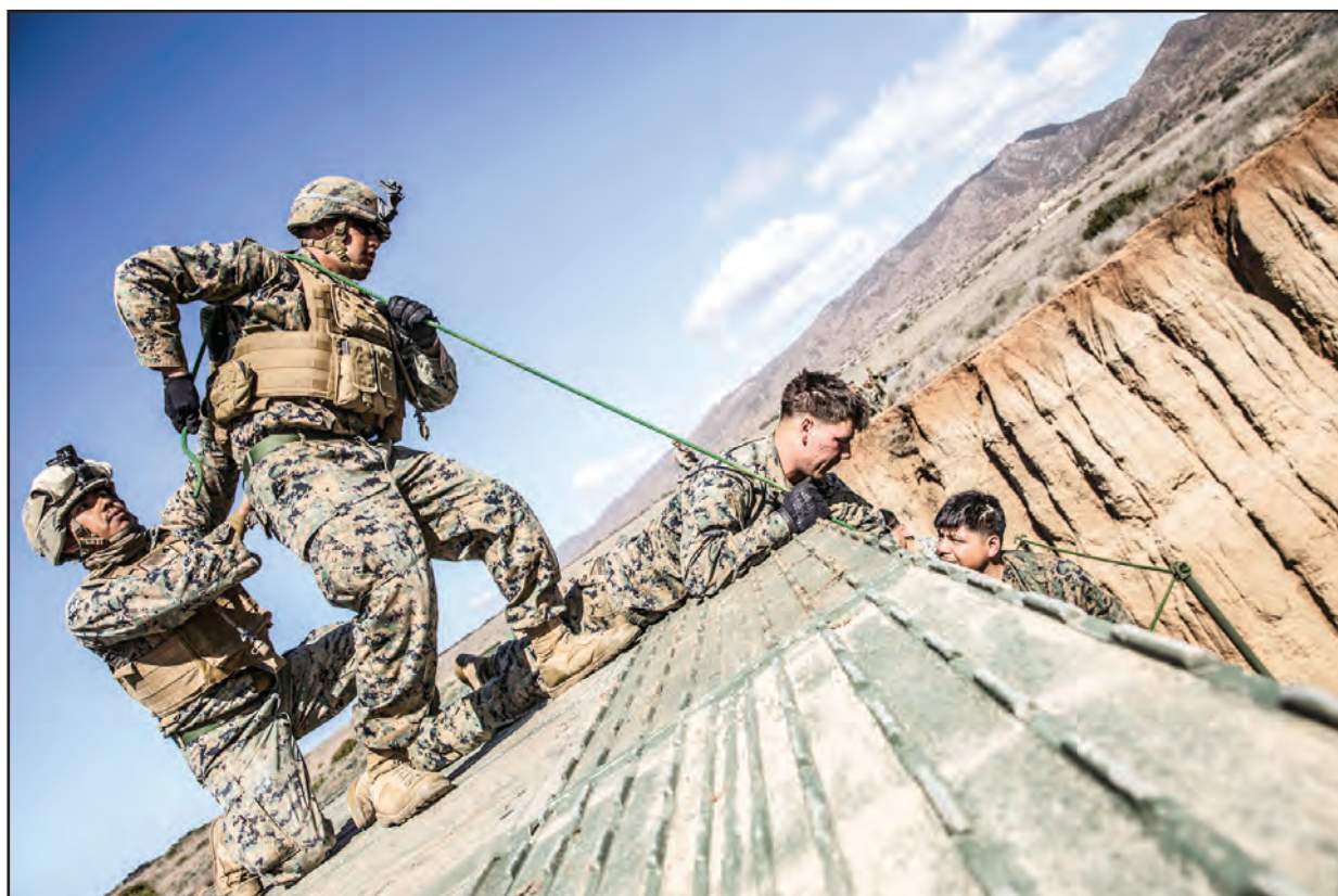
Marines with Bridge Company, 7th Engineer Support Battalion, 1st Marine Logistics Group, perform preventative maintenance to the medium girder bridge during a field training exercise at Camp Pendleton, Calif., Feb. 28. The Marines attach ropes to link reinforcements under the bridge to ensure it is tightly secured and in place.
